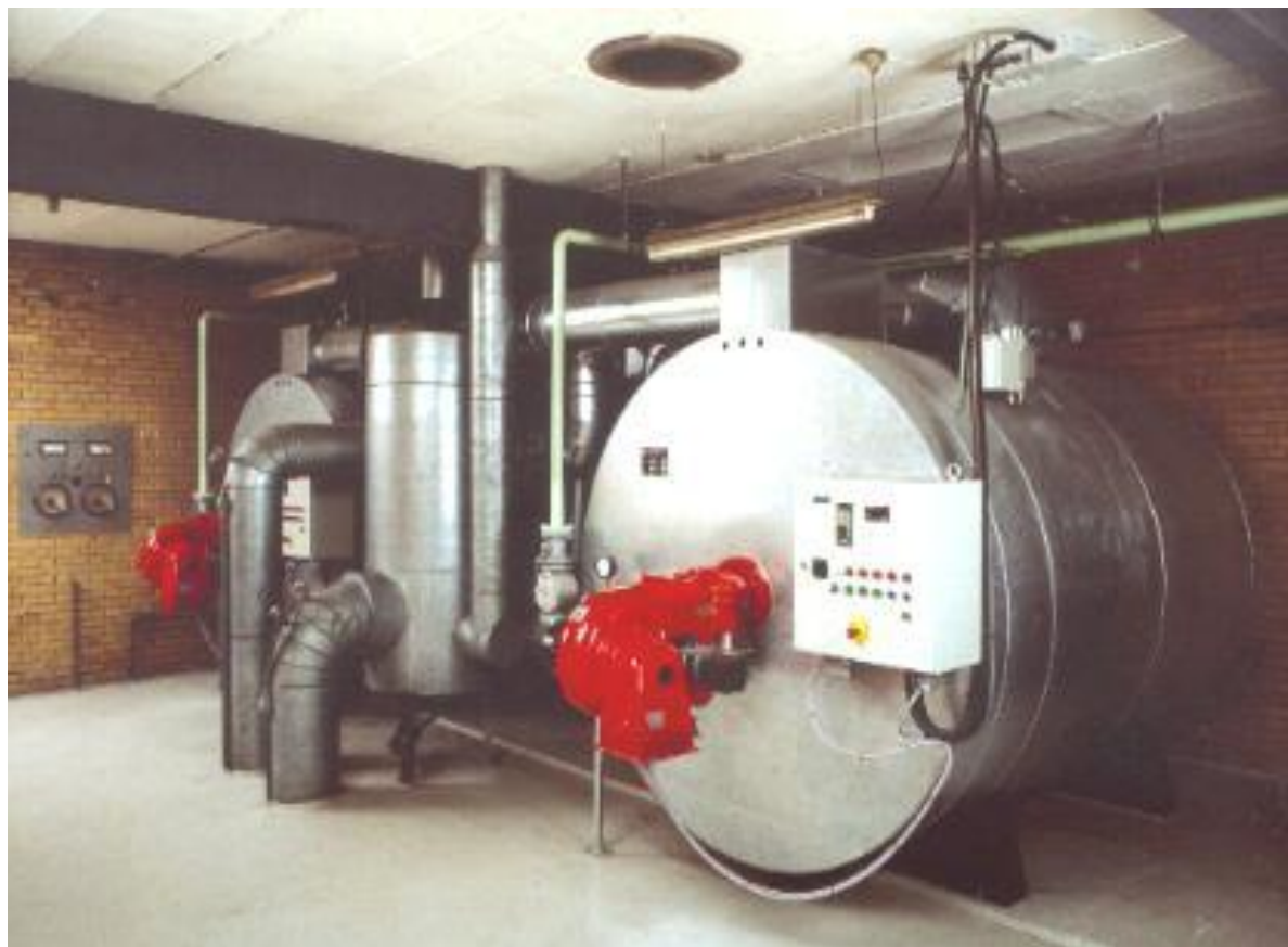
Fuel fired HTO - Process air heat exchanger
